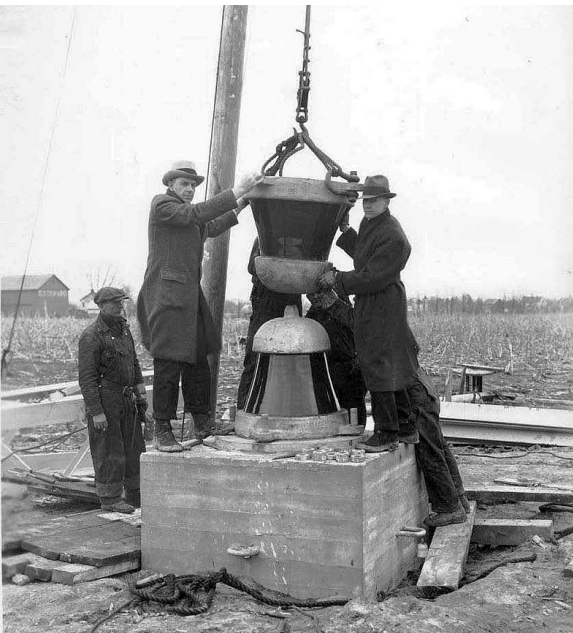
Setting the base insulator in place for the Blaw-Knox tower, 1933. The total weight on the insulator was about 450 tons.
