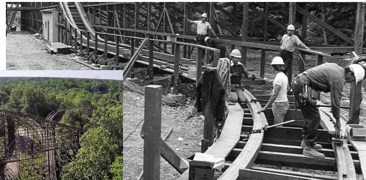
Construction of the, as yet un-named coaster in 1979. After hearing construction workers refer to building the coaster as a "beast of a project," park executives knew they'd found their name.
